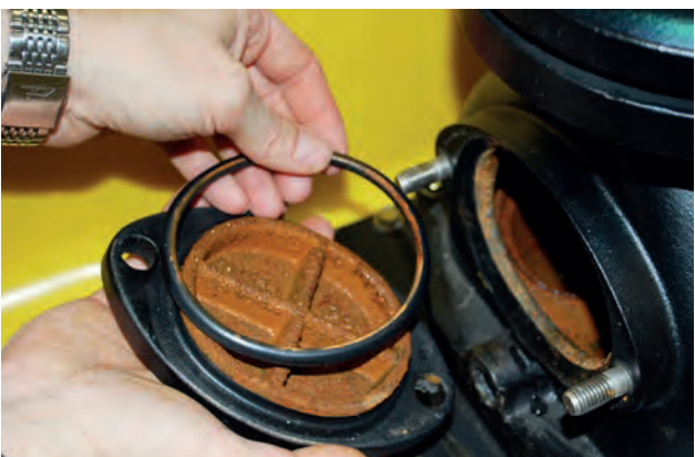
▶ Checking and cleaning the swing-type check valve
